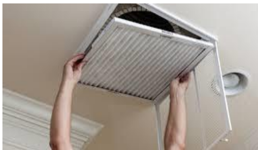
Filter in ceiling
