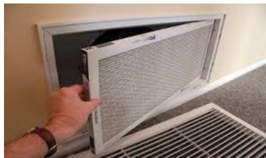
Filter in wall
