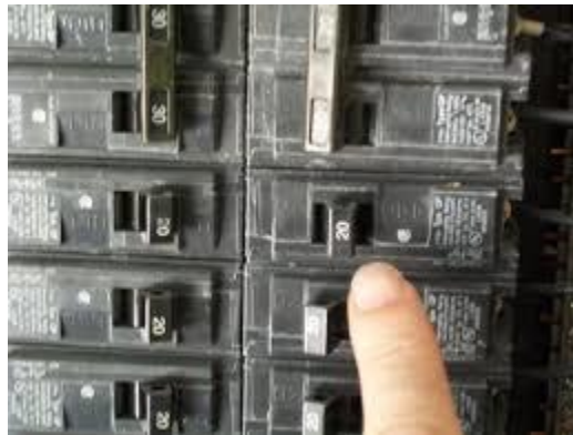
Reset Circuit Breakers
