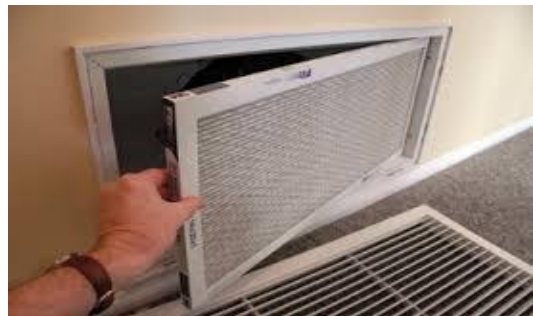
Filter in wall
