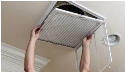
Filter in ceiling
