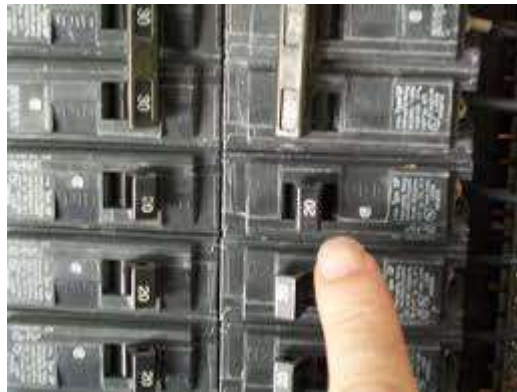
Reset Circuit Breakers
