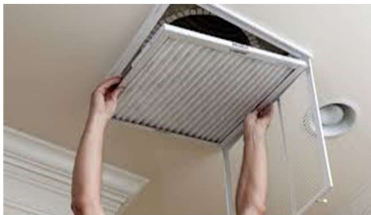
Filter in ceiling
