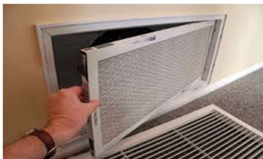
Filter in wall
