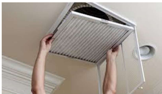
Filter in ceiling
