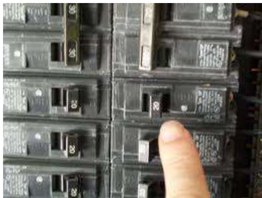
Reset Circuit Breakers
